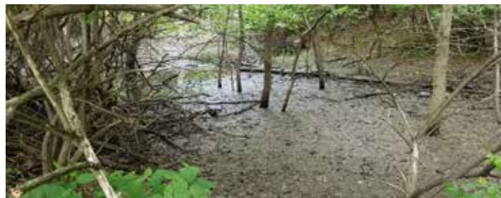
Compromised detention pond
